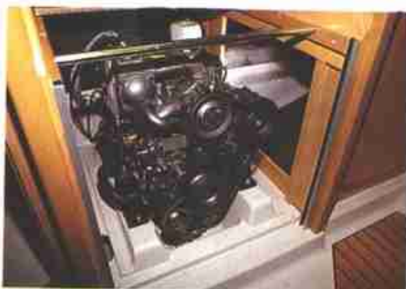
With the steps in place a substantial firebox surrounds the Yanmar 3GM saildrive unit
